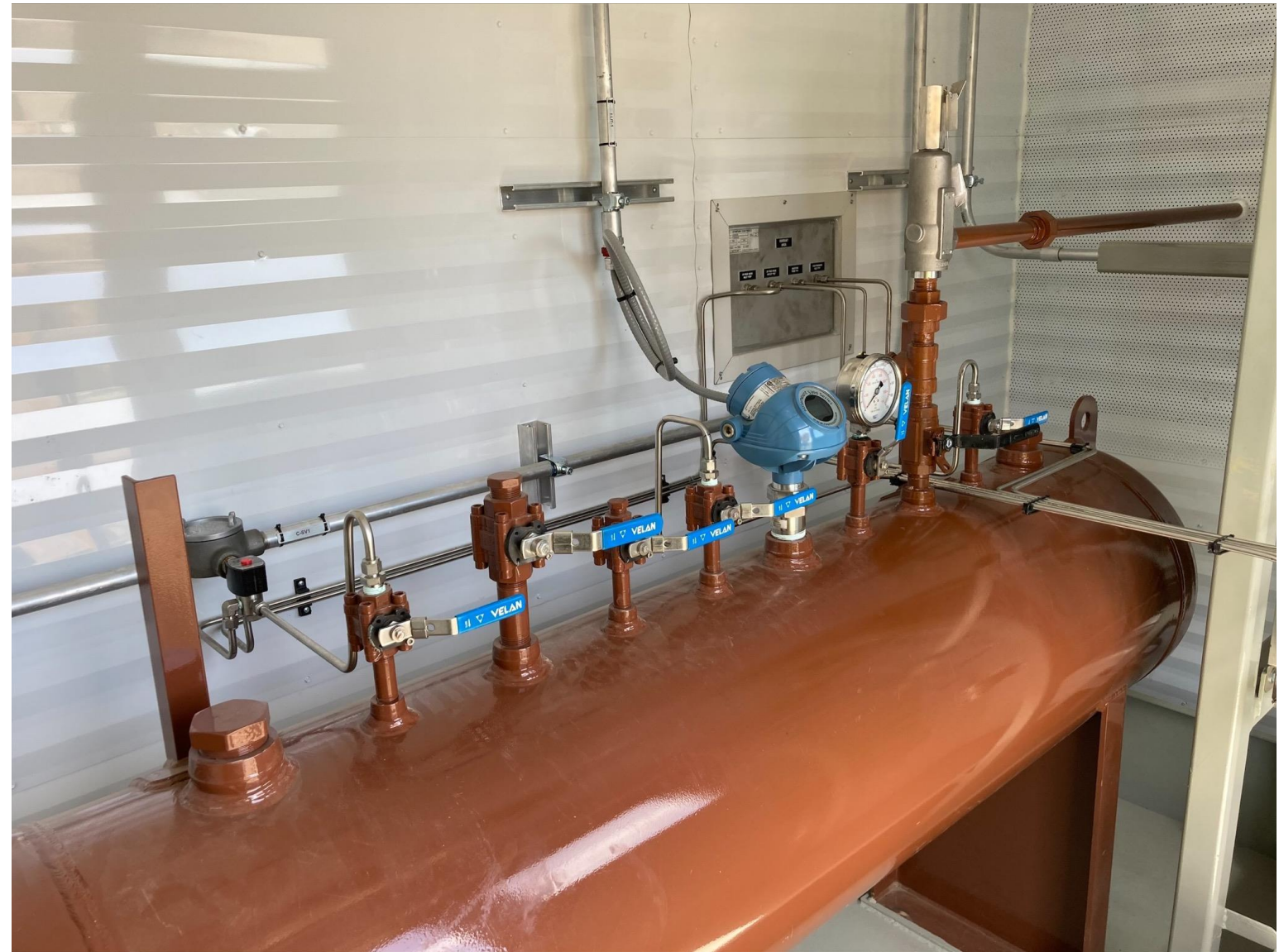
100 US Gallon Tank with Secondary Containment
