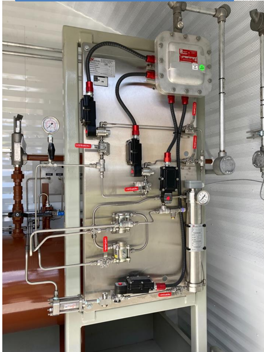
Dosaodor Odorant Injection System
